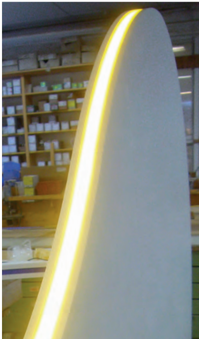
LEDs in Wandkante eingearbeitet LEDs installed into wall edge
